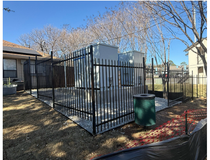
Shadow Brook Resilience Hub, battery storage system Holistic Energy Solutions
