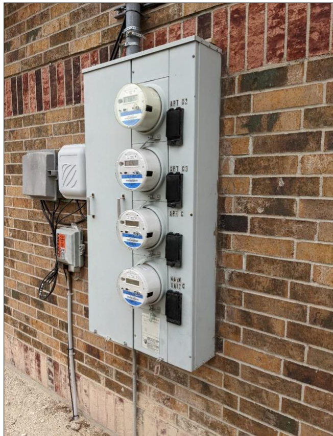
Figure 6. Building C meter bank—note additional meter for common area loads. Left side of panel is locked by the utility.
